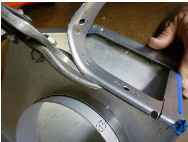
Figure 3: Shows a hole drilled in the corner and the flange of the stock box being cut away.
